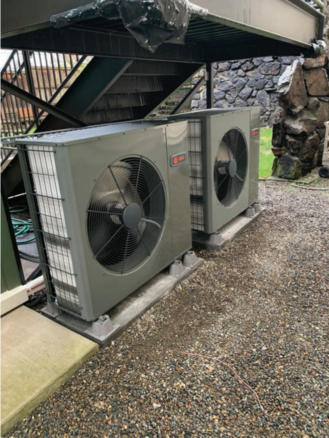
Heat pumps at the Tacoma Program Center.
